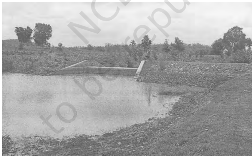
A small dam
