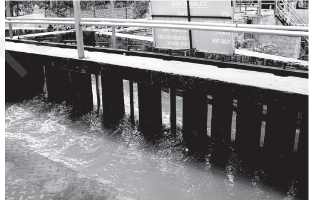
Fig. 18.4 Grit and sand removal tank
